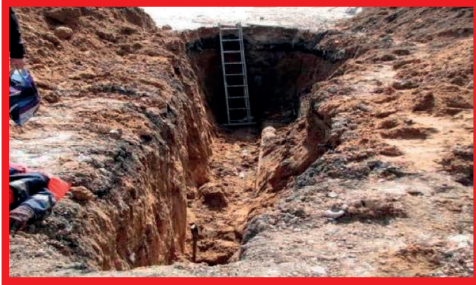
Fatal Accident 2009: Trench (2.1m) collapsed no shoring/support.
