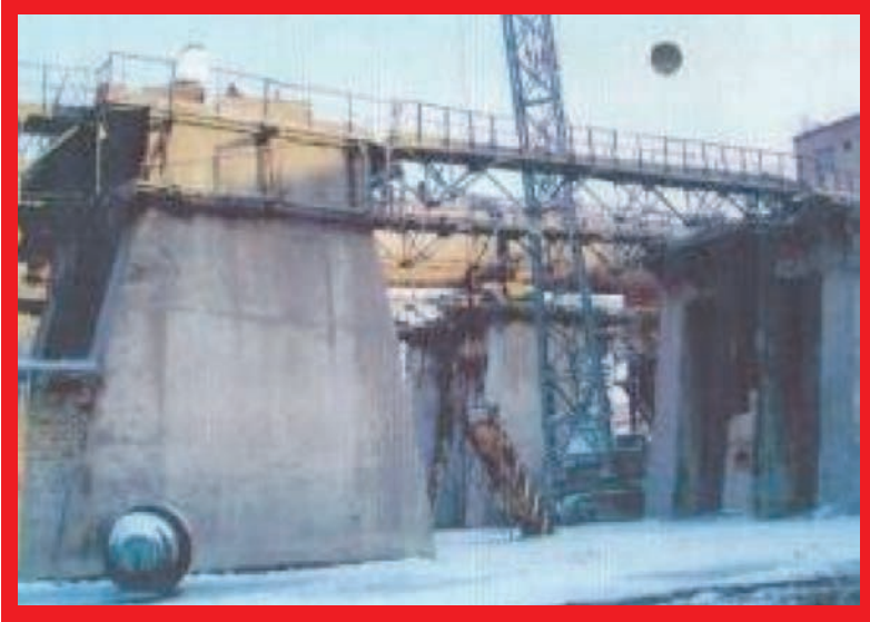
Group Fatal Accident - Case Study 2005: Contractor fell from walkway as it was being lifted.
