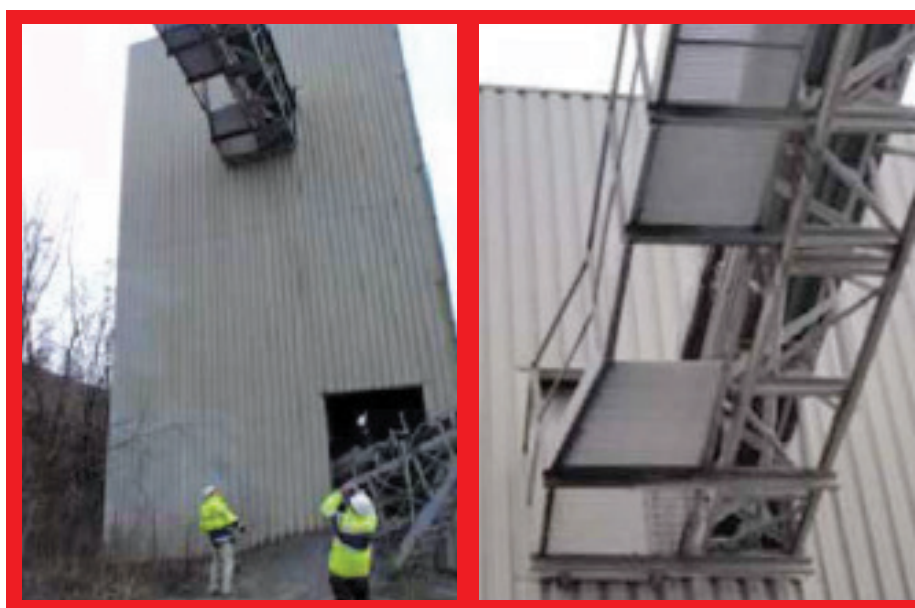
Fatal accident (non CRH site): Worker fell 14 metres when a section of walkway grid gave way. The grid securing bolts had become loose, over a period of time, due to the nearby vibrating screen.
