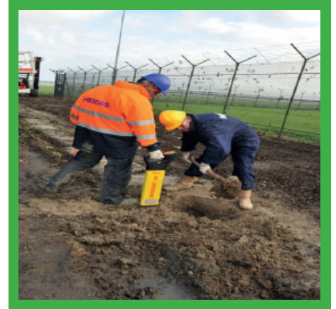
Checking for the presence of underground services prior to the erection of fencing.
