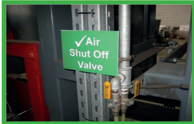
Clearly identified pneumatic isolation point.
