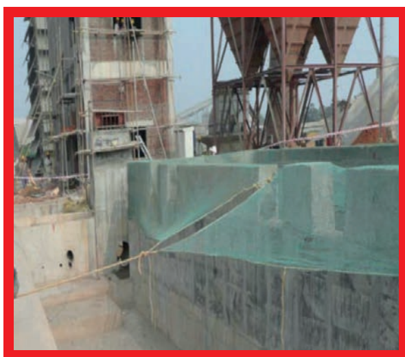
Fatal Accident 2011: Construction Project: contractor fell while crossing a wall during the construction of an extension.
