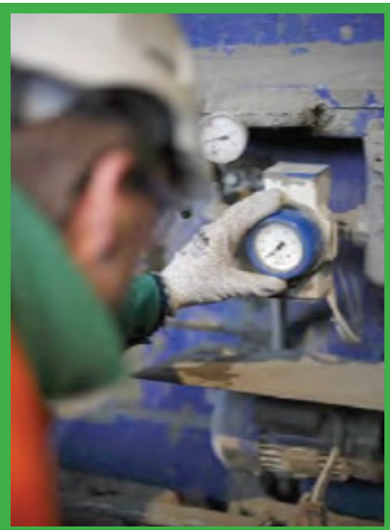
A confirmation check that all residual air has been vented from the system.
