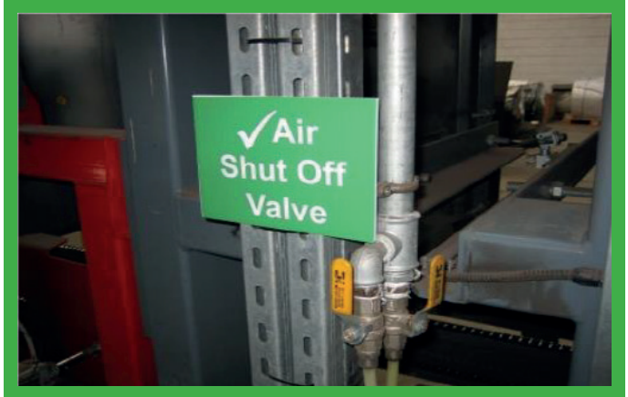
Clearly identified pneumatic isolation point.
