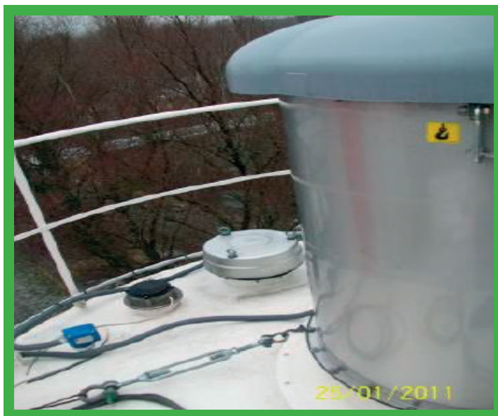
Last line of defence: Filter chained to silo structure.
