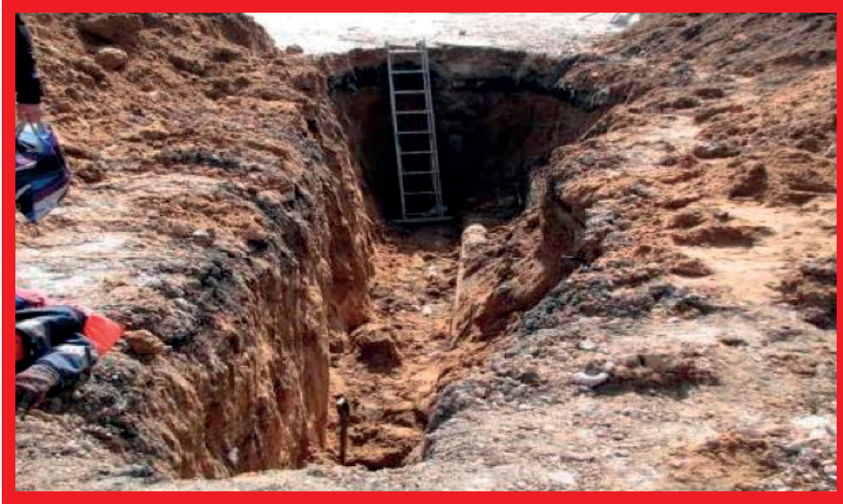
Fatal Accident 2009: Trench (2.1m) collapsed no shoring/support.
